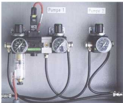
Controllers for the system pressure
